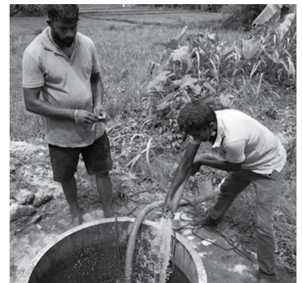
Hingalgoda, Halwitigala and Kurupanawa Tea Factories conducted a well cleaning Programme to clean over 29 wells which were flooded
